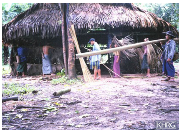
Villagers from K--- village in Dwe Lo Township, Mu Traw District doing ‘loh ah pay’ for the SPDC in July 2002. An officer of LIB #365 (under Battalion Commander Chit Nyo) ordered them to build this storehouse for the battalion’s rice and other foodstuffs. The photo was taken in July 2002. [Photo: KHRG]
