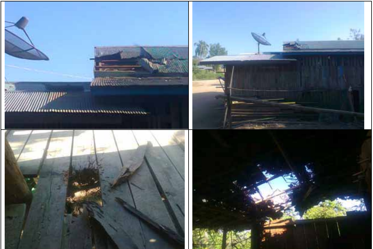
The photos above were taken on December 15 th 2010 and document examples of damage to property caused by indiscriminate firing of heavy artillery in Waw Lay village. Waw Lay has been one of the focal points during the current conflict in eastern Dooplaya. Waw Lay villagers have been endangered both by the unstable security and military situation and the reckless use of weapons by soldiers in the area. KHRG reported fighting in Waw Lay on December 13 th and 14 th 2010, with more than 20 shells reported to have landed in the village between 1:00 – 1:20 pm on December 13 th 2010. [Photo: KHRG]
