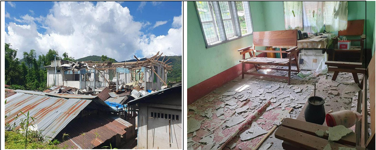
These photos were taken in July 2023 in B--- village, Htee Thar Saw village tract, Daw Hpa Hkoh Township, Taw Oo District. They show a Roman Catholic nunnery destroyed by the SAC air strike on July 22 nd 2023. [Photos: Local villager]
