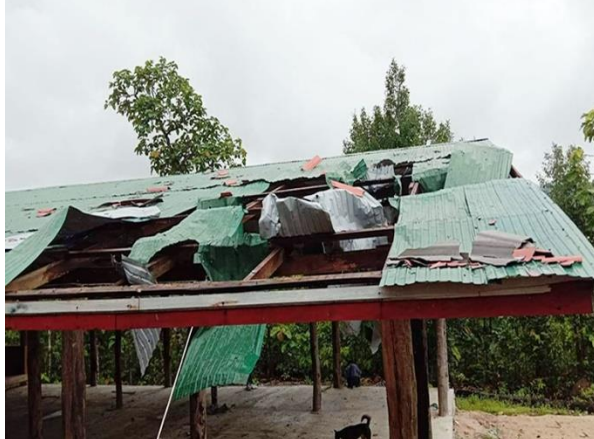
These photos were taken on May 18 th 2022, right after an SAC air strike in Thay Baw Boh village, Thay Baw Boh village tract, Kaw T’Ree Township, Dooplaya District. The photos show the damages to the local church and hall. Church property, including a piano, an amplifier and a guitar were also damaged by the attack. [Photos: Local villager]
