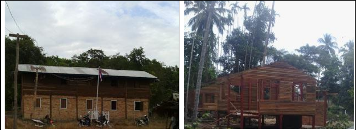
These photos were taken on January 10 th 2017 in Htee Lay Hkaw village, Pa Yah Raw village tract, Bilin Township. These photos show a college and its building established by the Thaton District [authorities], including the construction of teachers' houses. This place located in foot-hill near Htee Lay Hkaw village.
