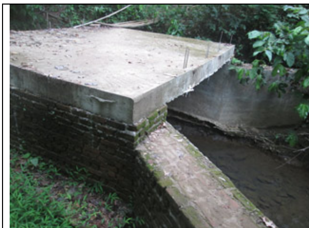
This photo was taken on June 22 nd 2016 by a KHRG community member in Bu Tho Township, Hpapun District and shows the bridge that was constructed by the Burma/Myanmar government at Way Hka Lo River between Way Hka village and Htee Ber Hka Hta village without the permission of the KNU. They [the Burma/Myanmar government] also have a future plan to renovate it too. [Photo: KHRG]
