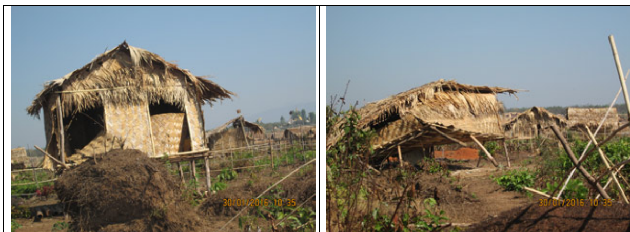
These photos were taken by a KHRG community member on January 30 th 2016, in the A---, Wa Da Kwin village, Moh Hk'Maw village tract, Kyaikto Township, Thaton District. The photos show villagers' houses that were destroyed by members of the local village authority. [Photos: KHRG]
