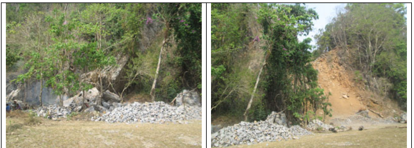
These photos were taken by a KHRG researcher on April 6 th 2013 in M--- village, Paw village tract, Paingkyon Township, Hpa-an District. They depict the cliff erosion next to Naw T---’s farm plot due to stone mining conducted by BGF Officer Lah Thay. [Photos: KHRG]
